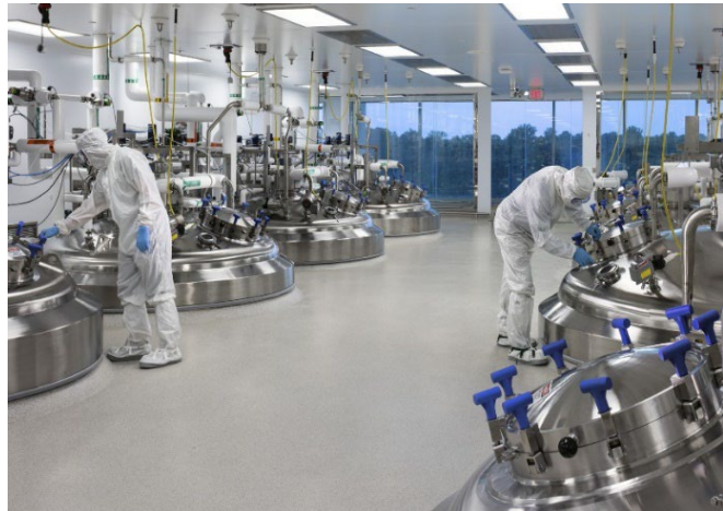
A manufacturing area in a GMP facility
