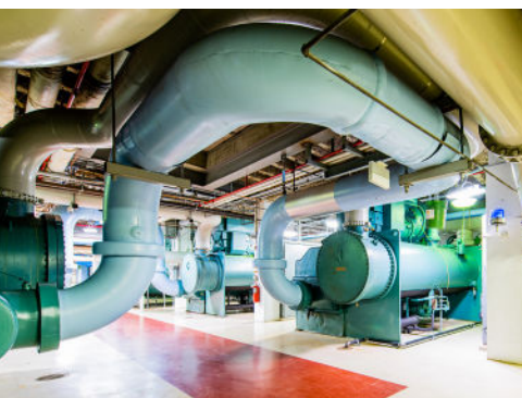
P3 District Energy: City of Cincinnati
